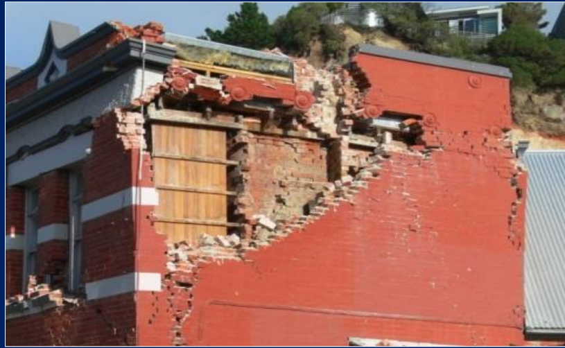
June 13, 2011 Magnitude 5.5 and 6.0 earthquakes
