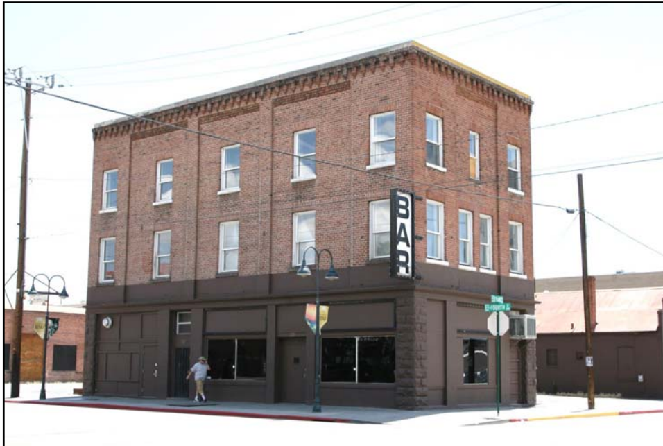
Three story URM with some earthquake cracks; occupancy is variable
